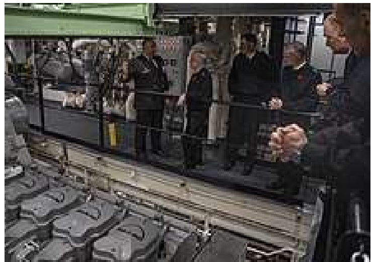
The Engine Room. 4 diesels at bottom left.
